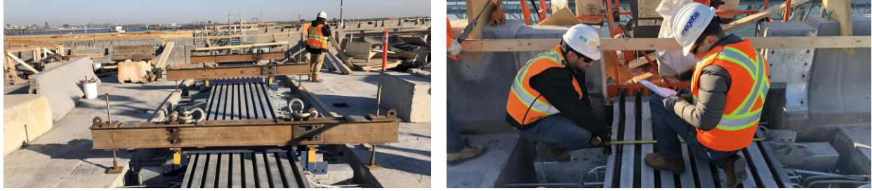
Figure 3: Installation of a 7-gap joint, ensuring proper pre-setting of width at time of connection to the main structure in order to ensure that all future movements can be properly accommodated
