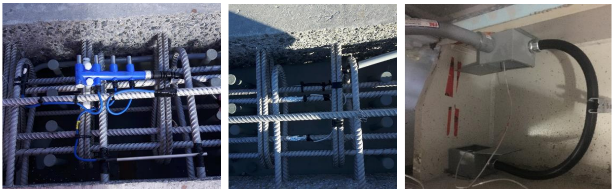
Figure 4: A corrosion sensor (left), and strain gauges of different types (center and right), as installed
